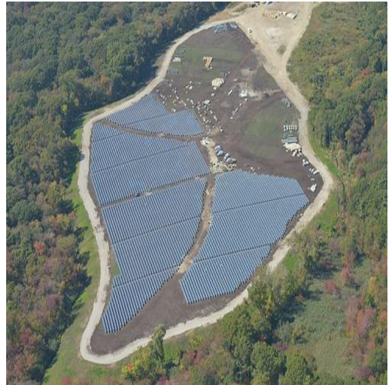
City of East Providence - 3.71 MW Solar Project
